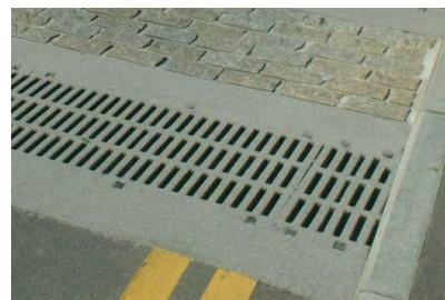
Non Slip Resin, and it looks and is safe to ride over
